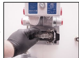
16. Check all leaders in the main socket. If bad conditions – replace the connection socket!
