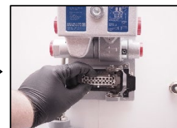
24. Check all leaders in the main socket. If bad condition – replace!
