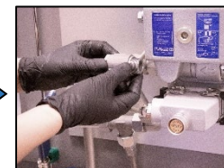
2. Remove the pipe from oil mist detector.
