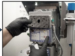
6. Clean the surface and replace the gasket for inspection cover.
